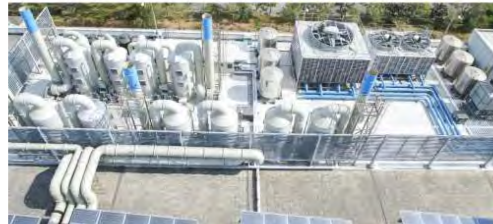
Continue to improve on the optimisation of energy conservation for our scrubbers, which are our single biggest user of electricity.
